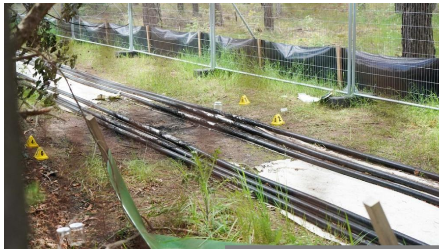
Six high-voltage cables supplying power to the site of a Tesla “gigafactory” were torched near Berlin, Germany in May 2021. Translated from the communique: “Our fire opposes the lie of the ecological car.”.
